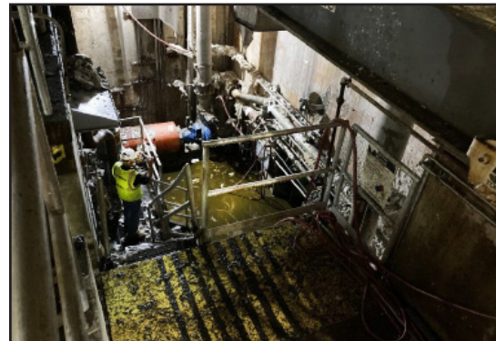
Previously, maintenance had to go down into this "pit" to adjust the packing.
